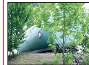
10,000 Gallon Fuel Tank
